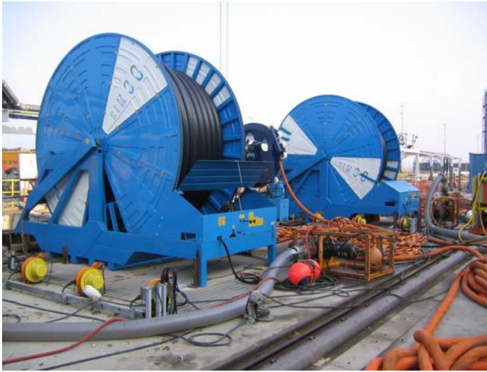
View on site of the five inch discharge hose reels
